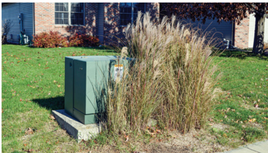
Do not plant shrubs close to padmount transformers or other utility equipment. We need at least 10 feet of clearance in front of the transformer.
